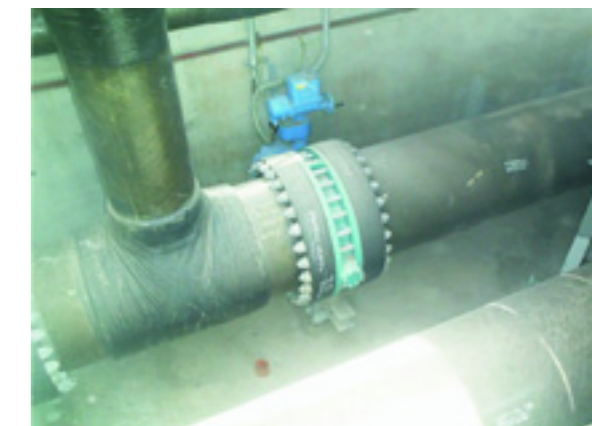
ND 54" AWWA CL.D, Flanged, POWER PLANT
